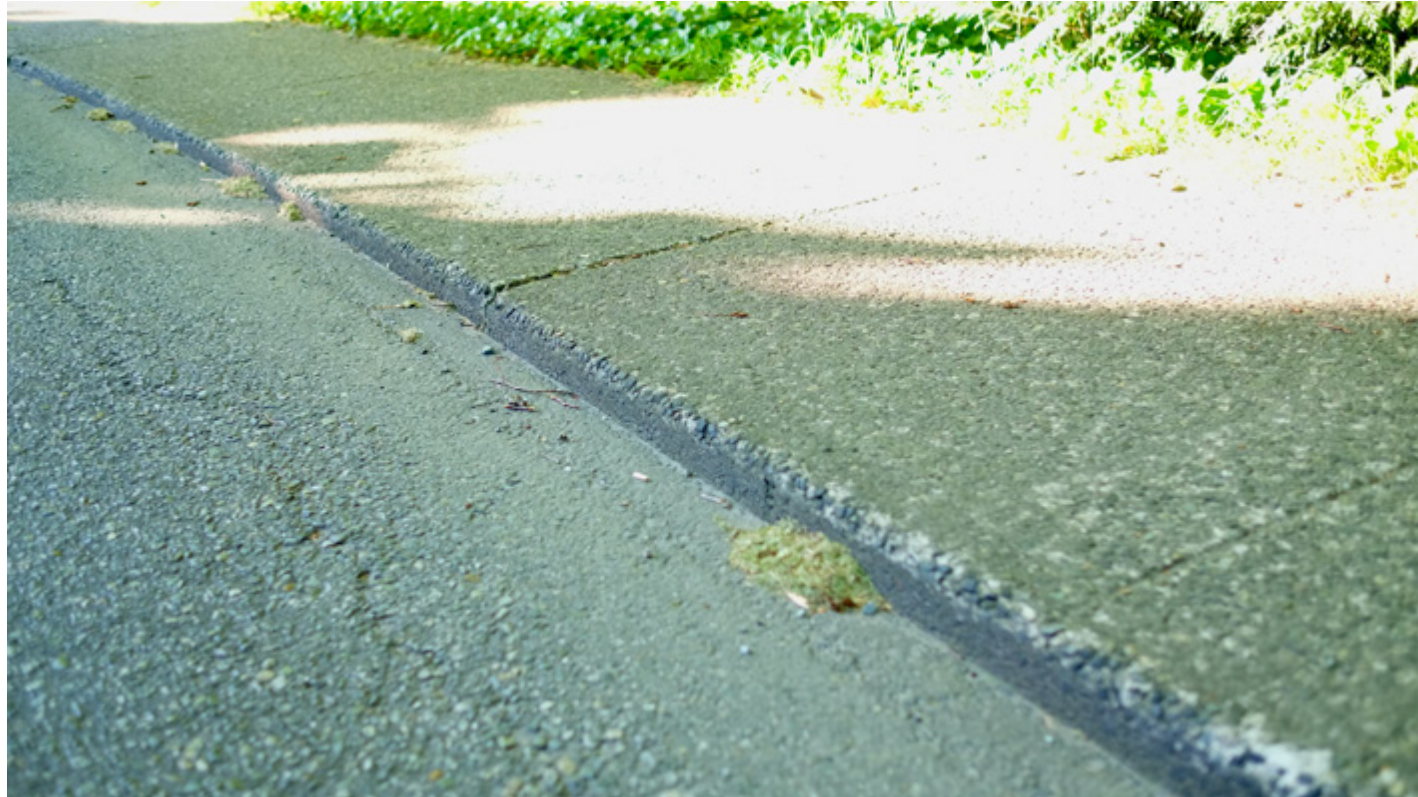
Insufficient curb height
